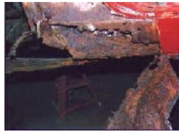
With the lower wing removed the full extent of the corrosion is revealed
