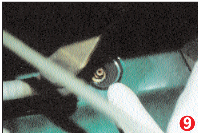
Bleed point two, at the heater, only visible when plastic cover is removed
